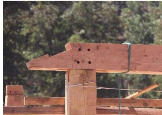
Scarf joint in the streak sill
