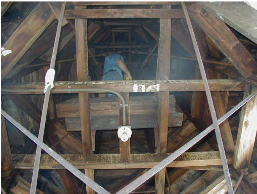
Steeple work is not for the faint of heart or for those with a fear of heights or bats
