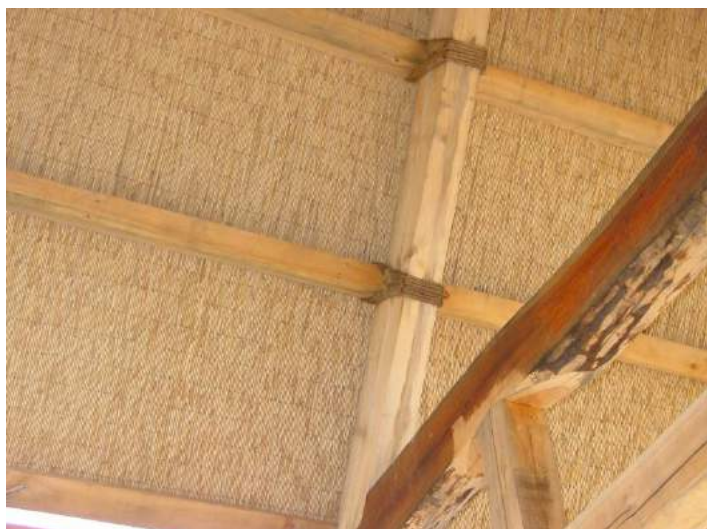
Japanese style timber frame with purlins lashed to the rafters; photo credit – Antique Barn Company
