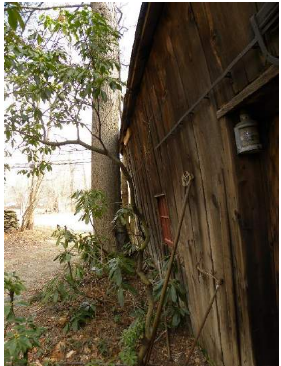
A sure sign that the tie beams were cut out
