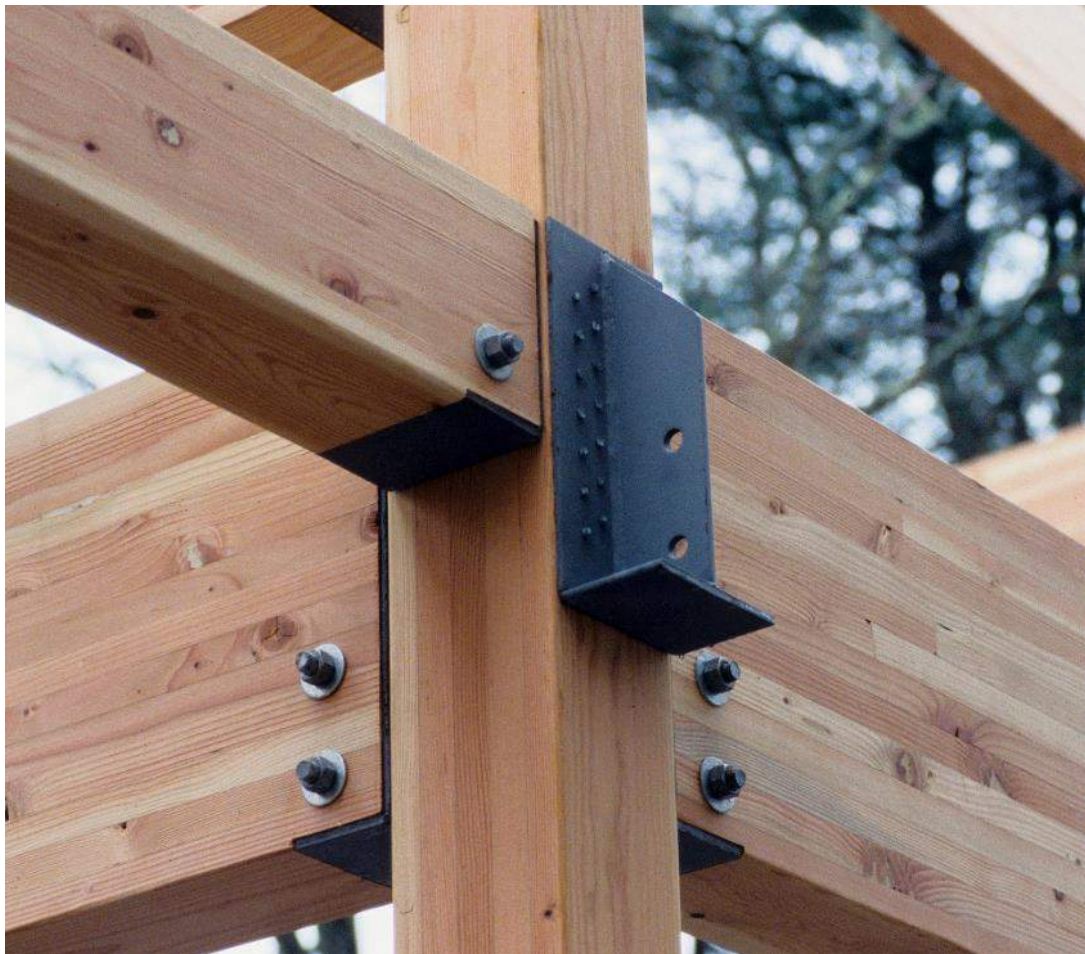
This stiffened seat connection is secured to the timber column with timber rivets
