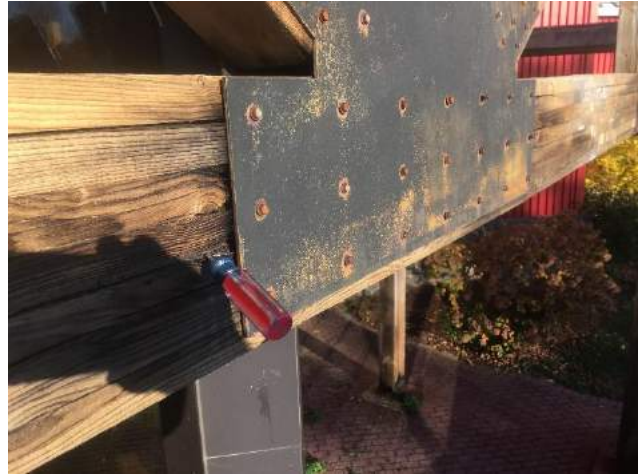
Fungal decay behind an exposed gusset plate
