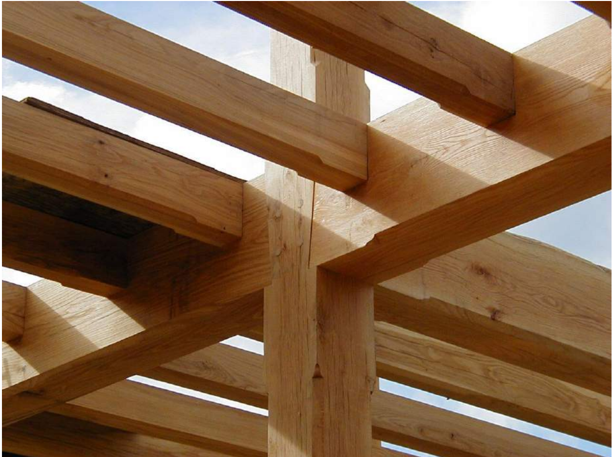
Chamfered timbers with ski tip stops on the joists and lamb's tongue stops on the posts and girders
